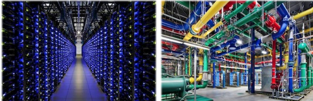
Figure 2 Inside Google's data centres
