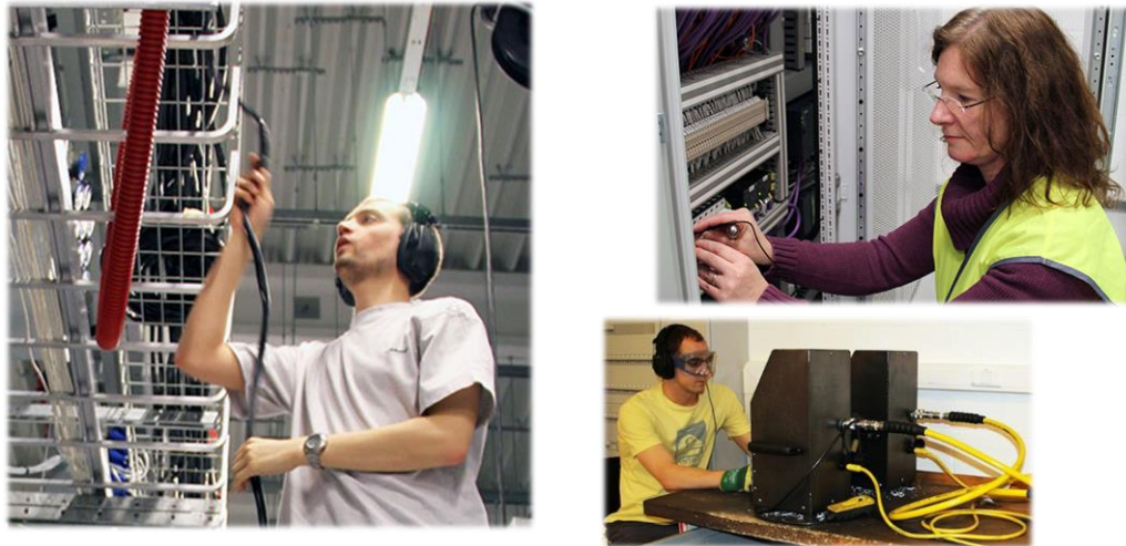
Figure 6 Working at the St. Ghislain–Mons data centre
