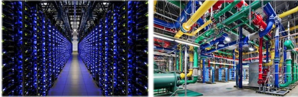
Figure 15 Inside a Google data centre
