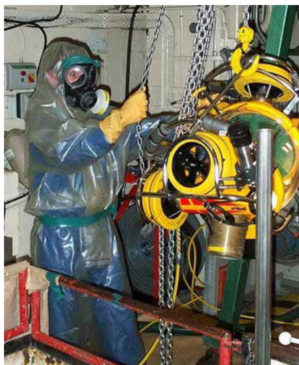
Using remotely operated vehicles to help in the cleaning up of legacy ponds and silos
